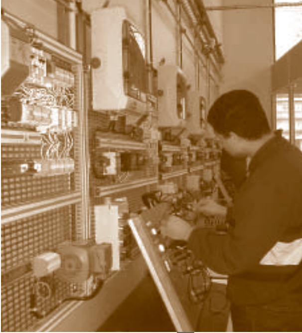
Electrical engineering facilities
